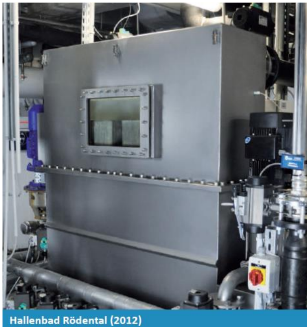
Figure 5. Filtration system using Saint-Gobain SiC dead-end filters in a public swimming pool in Germany.
