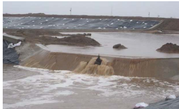
Figure 4: Surface runoff carrying huge silt
